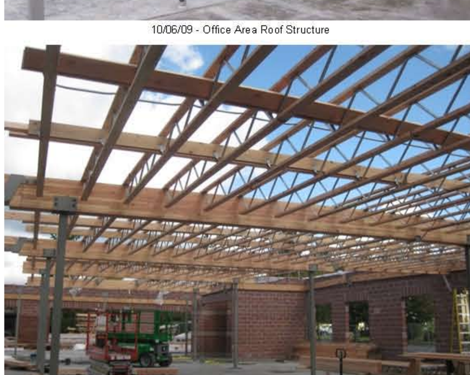
09/28/09 - T-JL's at Office Area
