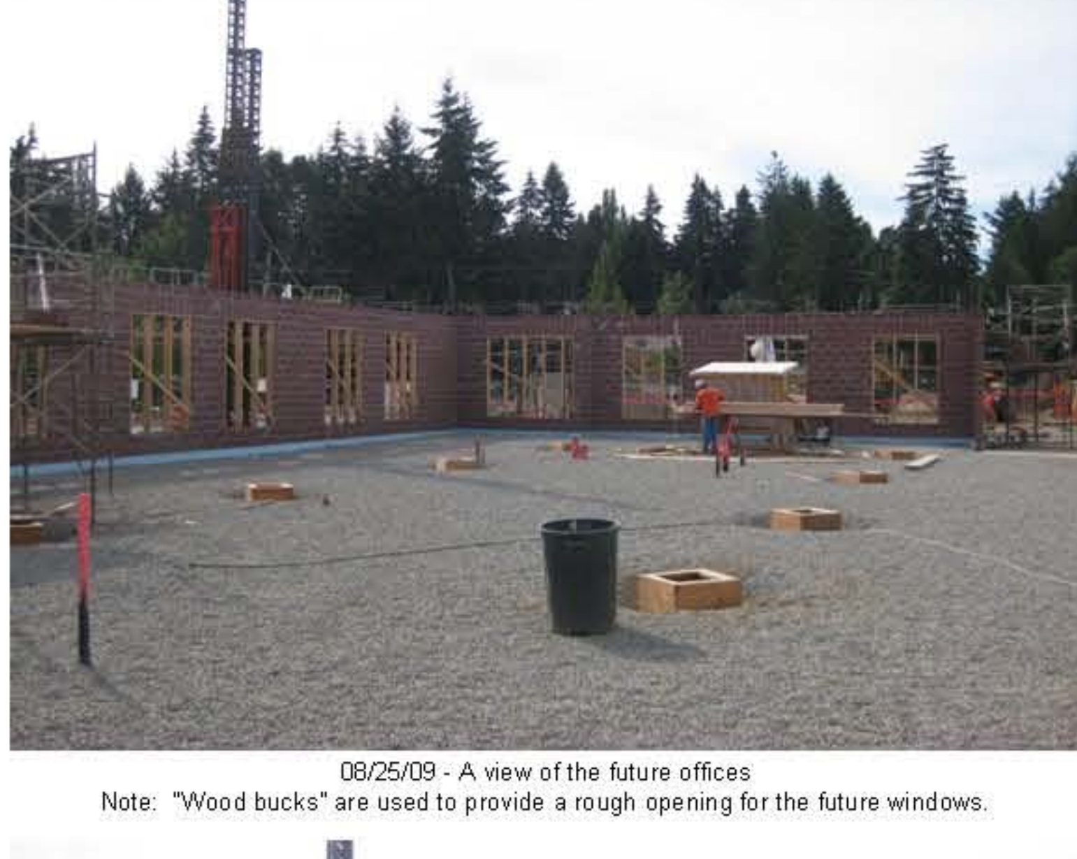
08/25/09 - A view of the future offices Note: "Wood bucks" are used to provide a rough opening for the future windows.
