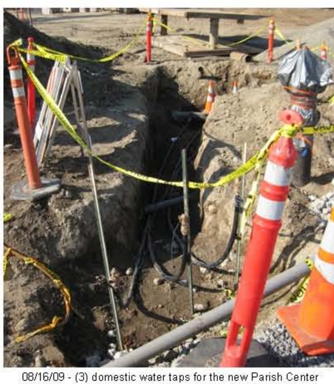
08/16/09 - (3) domestic water taps for the new Parish Center
