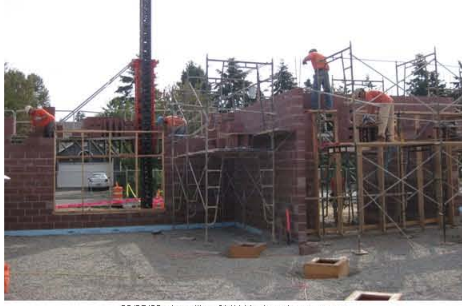
08/25/09 - Installing CMU block at the east entry Note: CMU block is installed and grouted in 4' increments. In this area they are on their 3rd lift
