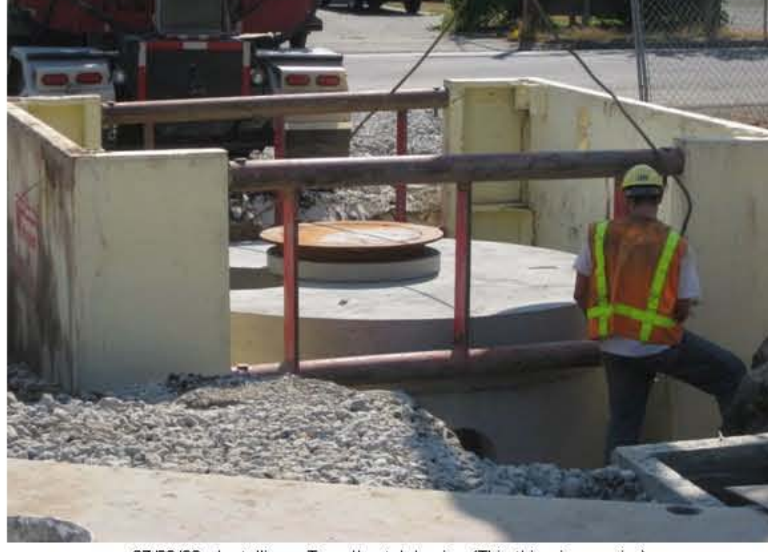
07/28/09 - Installing a Type II catch basin. (This thing is massive) It is for the new storm system and is located near our construction entrance.
