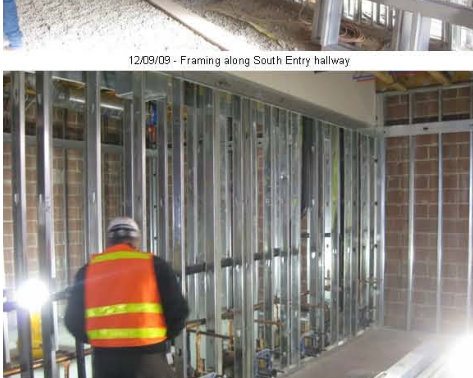
12/08/09 - Carriers for restroom toilets
