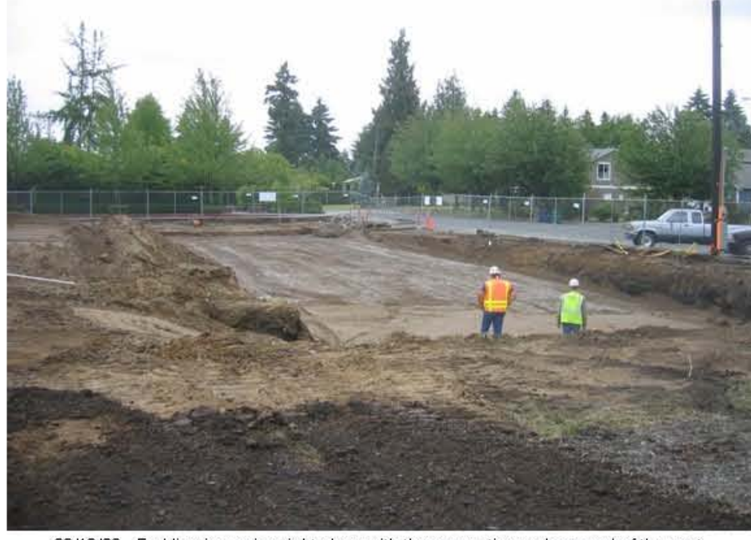
06/18/09 - Fruhling is moving right along with the excavation and removal of the peat.
