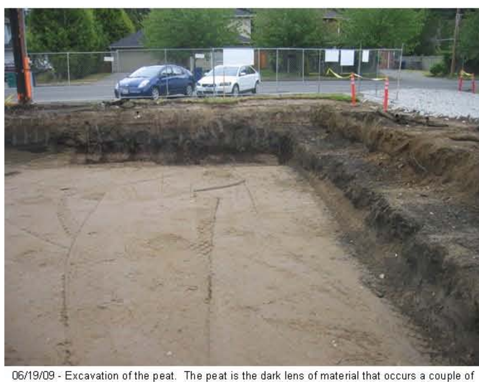
06/19/09 - Excavation of the peat. The peat is the dark lens of material that occurs a couple of feet below the top of grade.
